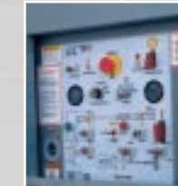
Base controls - override platform controls and permit operation from base for service and testing.
